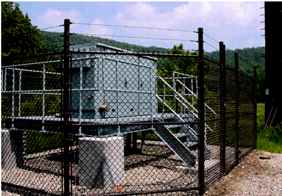
FIGURE 3-4 TYPICAL OUTDOOR ENCLOSURE CABINET ON RAISED PLATFORM
